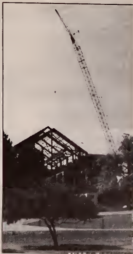
This photo of the approximately $11 million library/academic building under construction at Penn State Erie, The Behrend College, was taken in June. Since then, the roof has been installed and the front of the structure is bricked. The arched steel supports shown in this photo are covered, but the all-glass wall that will grace the building has not been installed. Completion of the brick and glass work is expected later this month.
